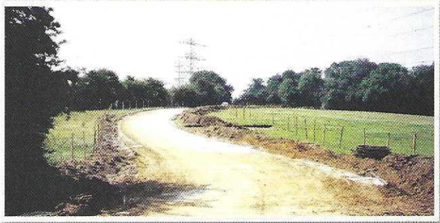
The special soil conditions on the temple land allowed us to use an old but highly effective technique of lime stabilisation and the road was well built in record time
